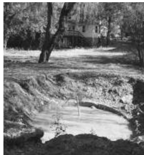
A test pit for a septic system is filled with water recently at 39-12 Douglaston Parkway, where DOB issued a stop work order September 15th. (The Douglaston & Little Neck Historical Society)
